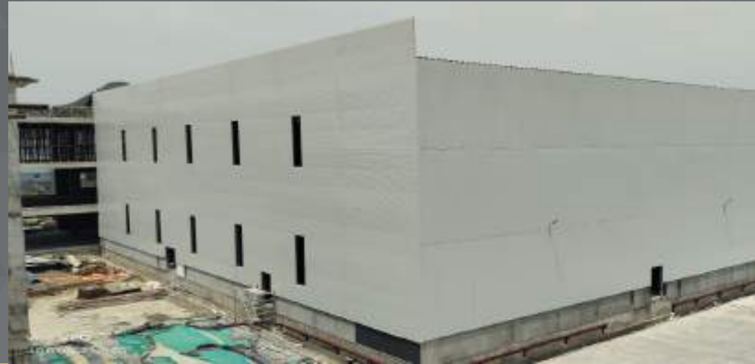
HVAC Ready : Cladding is done with PUR Sandwich Panels for Better Insulation and HVAC efficiency , also ensuring lesser Op-ex on Energy Costs
