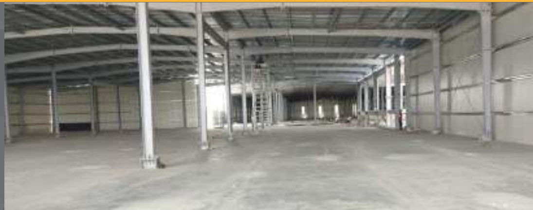
TR34 Rated Super Flat FM 2 Flooring : Ready for ESD and EPOXY application.
