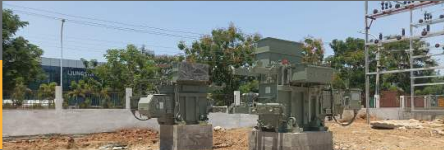
33KV 2500kva transformer core -02 Nos installation work completed and accessories will be installed after earthing work.
