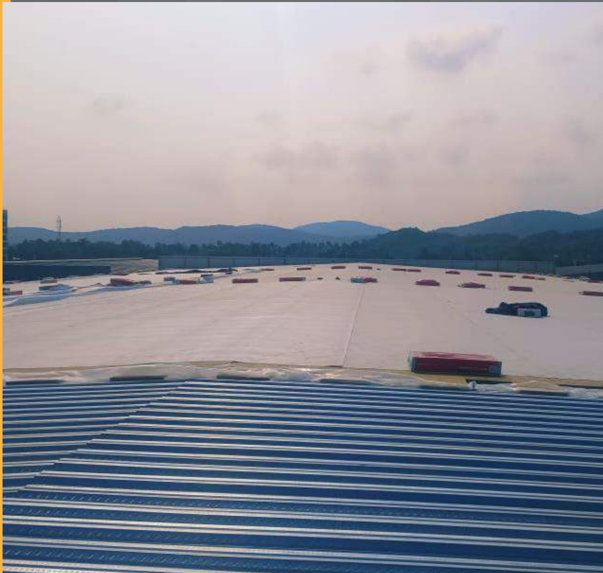
Leak Proof Roof : TPO Membrane + Rock Wool Insulation + Vapour Barrier + Deck Sheet (Ensures Zero Leak )
